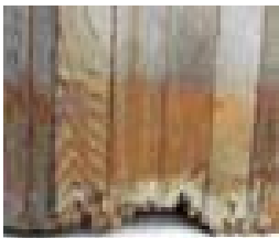
7 year-old spa with dry rot beginning to show, This spa had a thin plastic base over pressure treated 2x4 frame.
