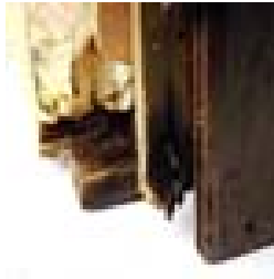
7 year old spa on pressure treated 2x4 base. The skirt is fine but the base is rotting from the inside out.
