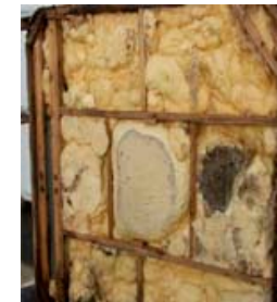
Spa bottom where the footwell rests on the ground to support the weight of the spa full of water and people.
